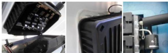
open junction box in the field poorly bonded junction box on the back sheet junction box with poor wiring
