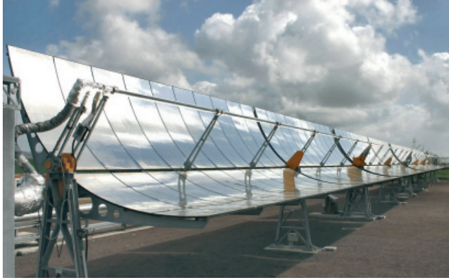
Figure 1 – CSP Parabolic Trough Solar Collectors
