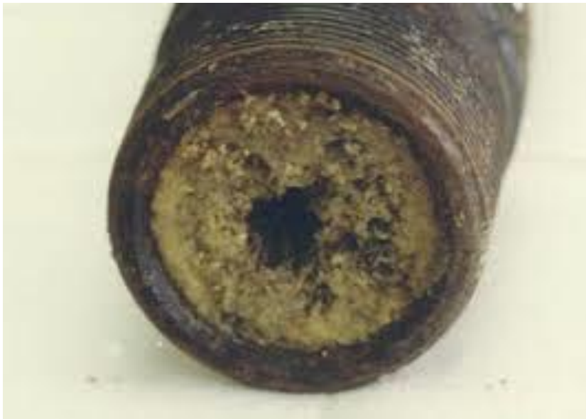
Figure 7. Blockage inside tubing by scale precipitation [3]
