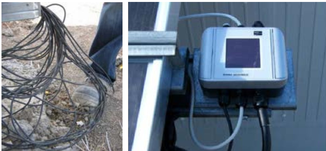
Figure 3.2. Examples of poor installation work
