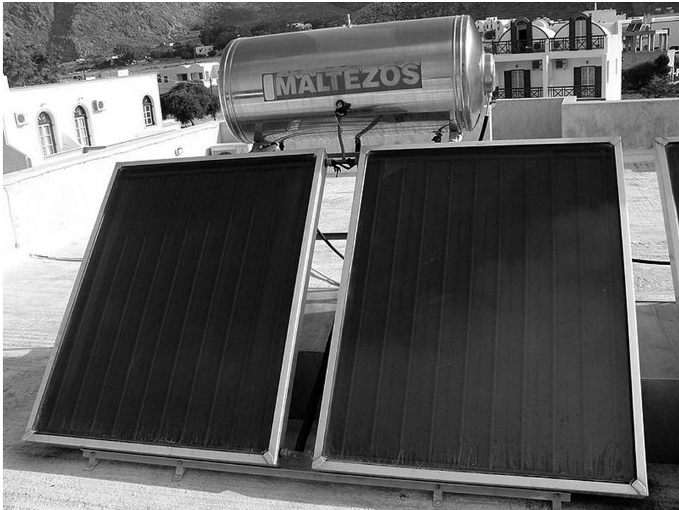
Figure 2.9 Solar thermal water heater on a residential rooftop.
