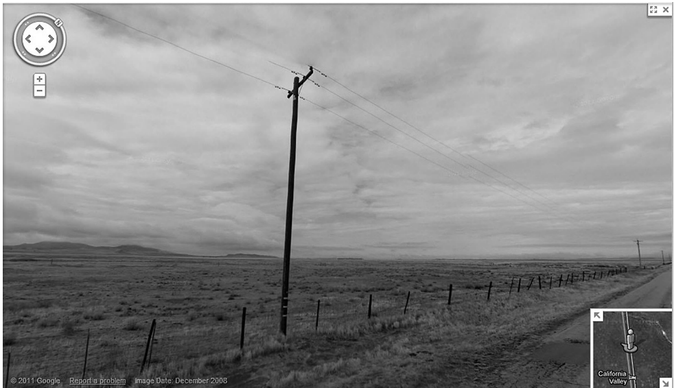
Figure 8.32 Screenshot Google Maps Street View showing transmission or distribution lines.
