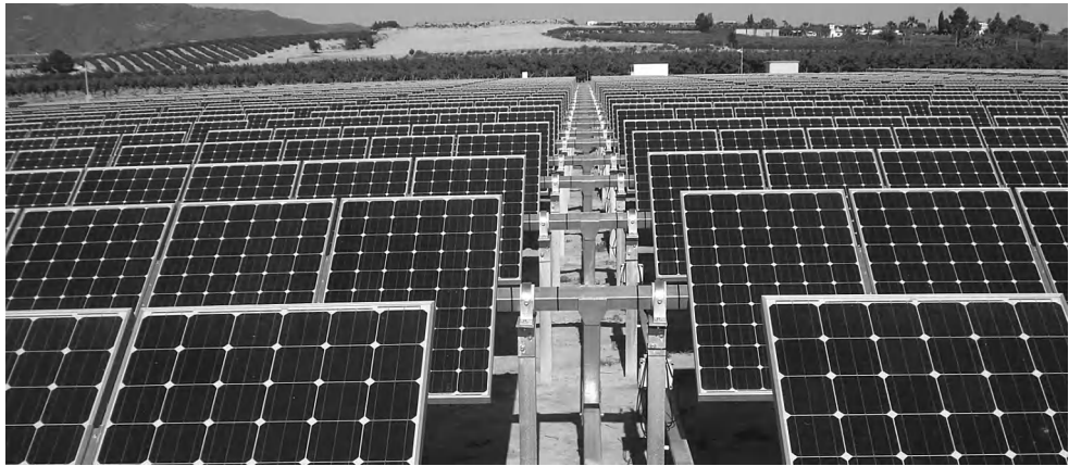
Figure 9.10 Horizontal SAT (Courtesy of PVHardware – Axone System).
