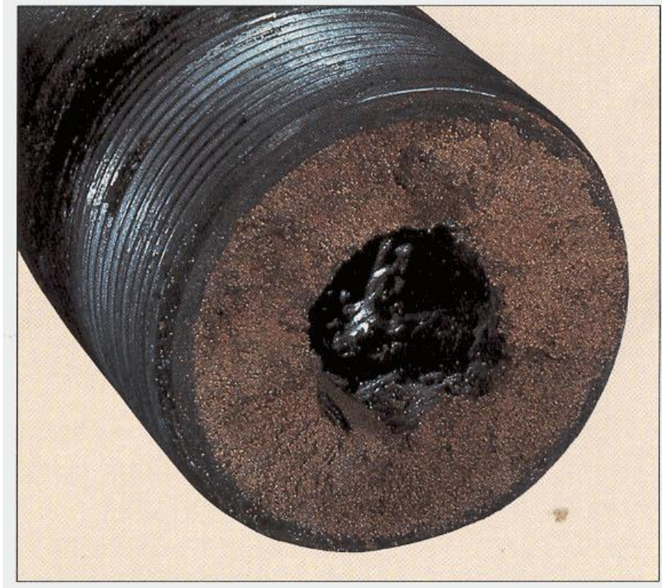
Figure 1. Asphalt-resin-paraffin deposits in the oil well tubings [1]
